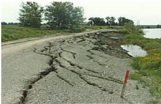
Failure of a road embankment
