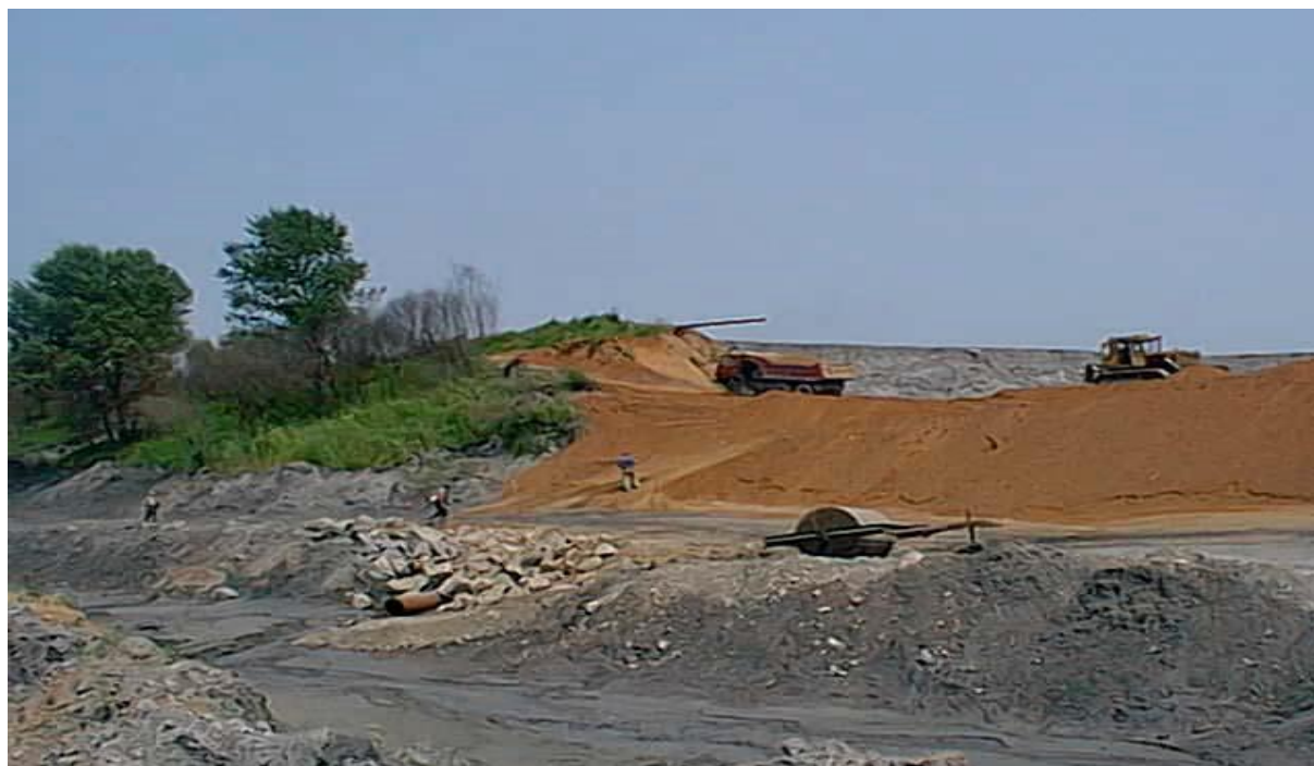
Fig.1.1 Breaching area due to failure of ash dam (Paul Robinson,Albuquerque,USA, )
