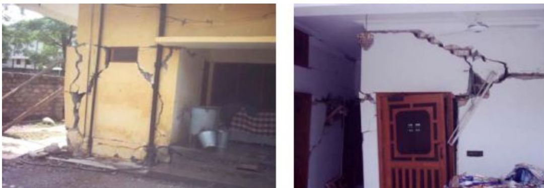
Fig. 1.1: Combined in-plane and out-of-plane failure mode in Kashmir 2005 (Naseer et al. 2010)
