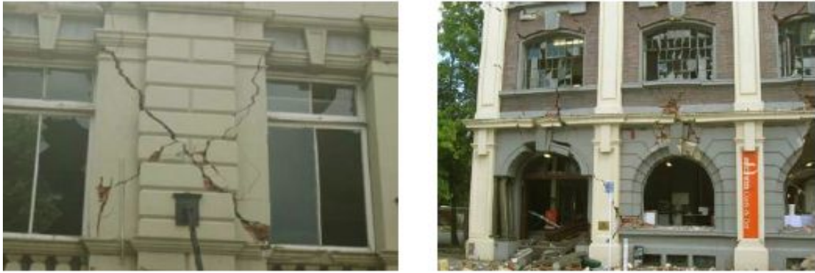
Fig. 1.2: Piers and spandrel failure (Ingham, 2011)
